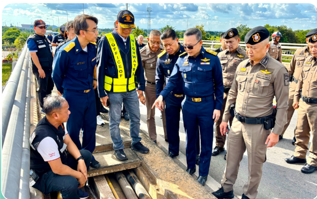
The field inspection in the area of the Second Thai-Lao Friendship Bridge in Mukdahan Province, to inspect illicitly installed data cables for distributing signals into the neighboring country
